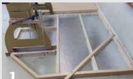
1 Subfloor effectively lowers the lathe height and provides a hidden chase for wires and an air hose. Foil-backed insulation helps keep feet warm.
